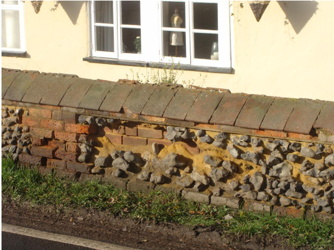
Picture 24. Wall to front of Hermitage Cottage in need of repair.
